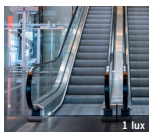
Escalators to enable users to safely disembark
