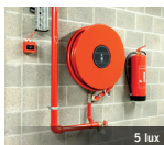
Near each place of fire-fighting equipment
