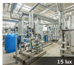
Plant rooms for generators and control equipment
